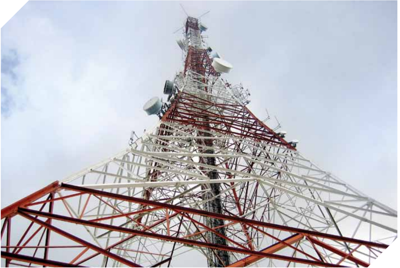
VIOM NETWORKS LIMITED FINANCED BY IDFC IS INDIA'S LEADING INDEPENDENT TELECOM TOWER COMPANY WITH A PAN-INDIA PRESENCE SPANNING ALL CIRCLES
